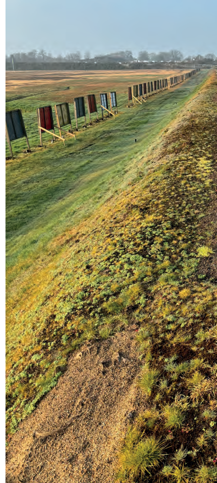
Above: Re-profiling of the mantlet, with the addition of over 140t of soil. Below: Replacement of all range floor pegs.
